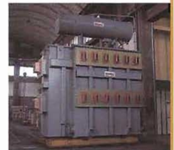
One of two rectifier transformers 2x22.6/32 MVA (Korea)
