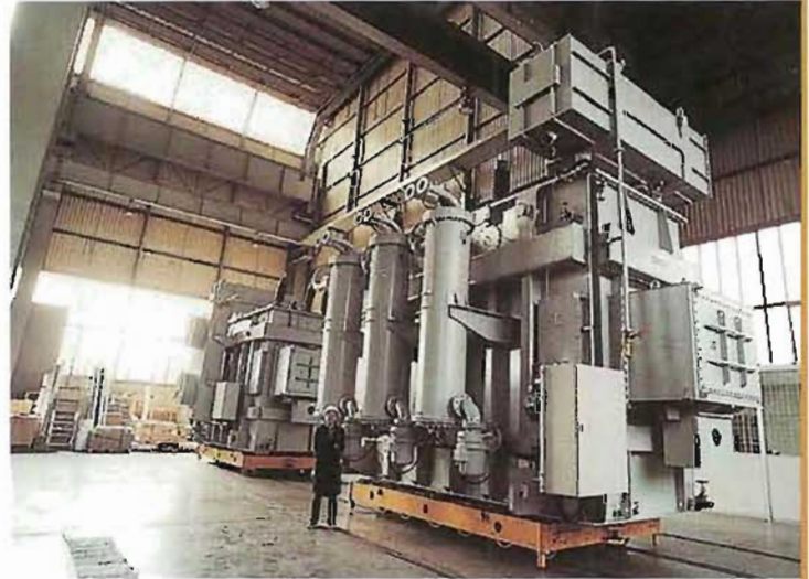
140 MVA EAF transformers 69/1.7 kV and a 82 MVA series reactor (USA)
