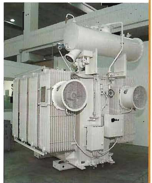
Mineral oil filled transformer - 9500 kV/6 kV
