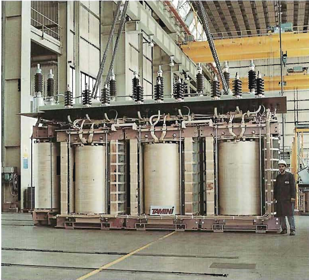
Internal view of a saturable reactor for a 123 MVA EAF transformer (France)
